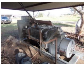
180kva Generator – Volvo Motor.
